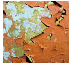
Chipped lead paint
